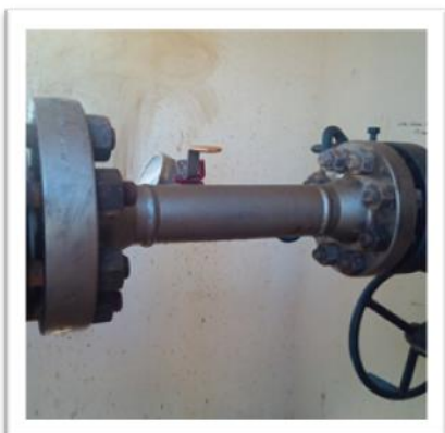
Application: Spool coated with InnoGUARD™ Environment: Produced water (70% chlorides) In service: 3+ years when photo taken
