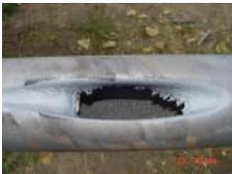
Hole Blasted Through Pipe
