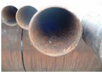
Severe Storage Pitting
