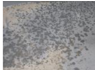
Water Staining on Floor of Sandblasted Tank
