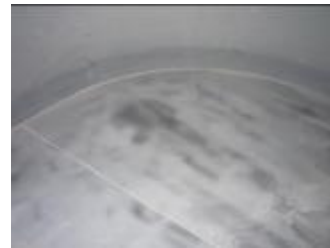
Mill Scale on Floor of Sandblasted Tank
